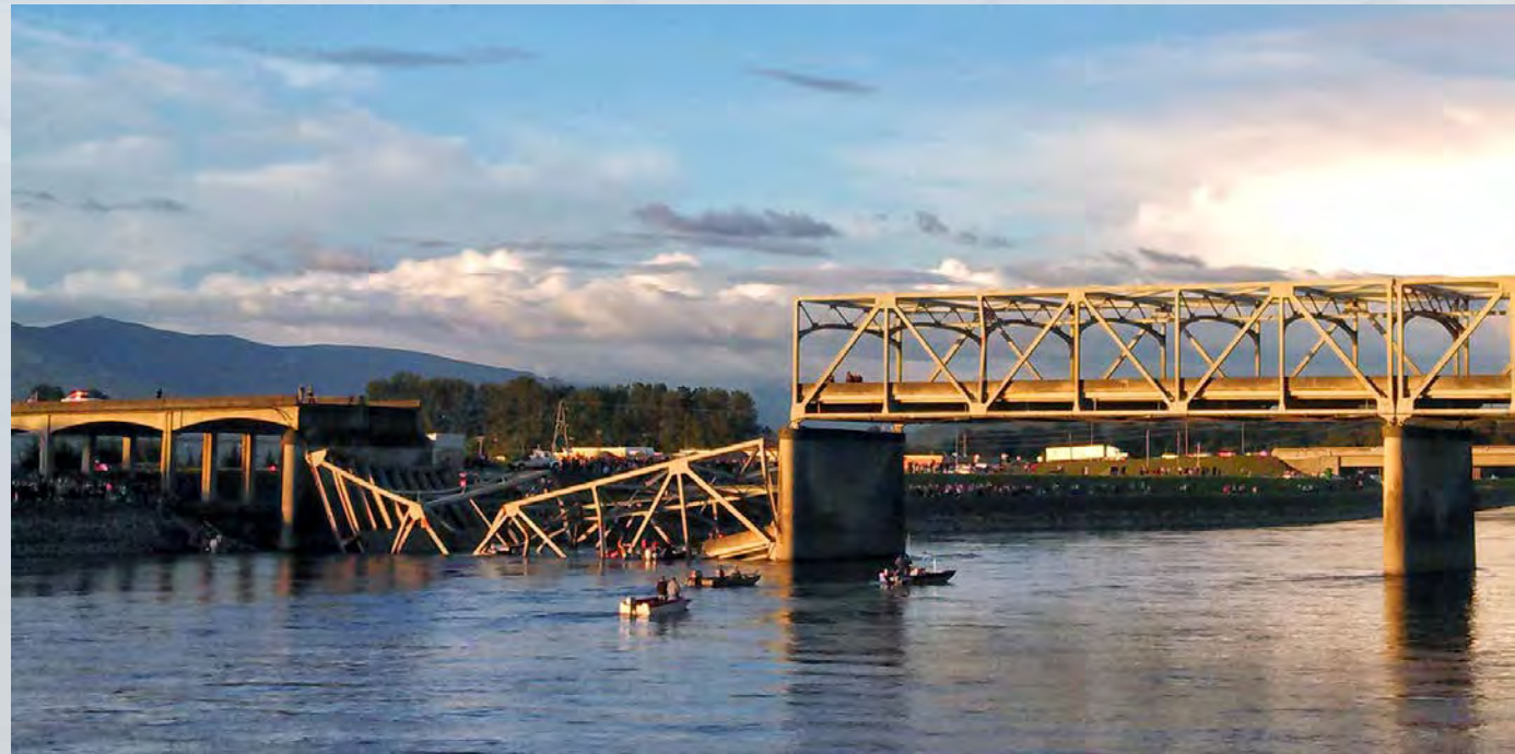
Skagit River Bridge failure caused by collision
