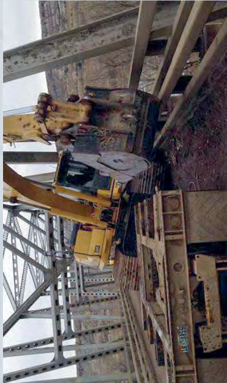
Long X Bridge collision
