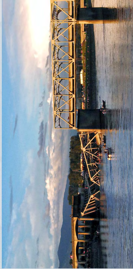
Skagit River Bridge failure caused by collision
