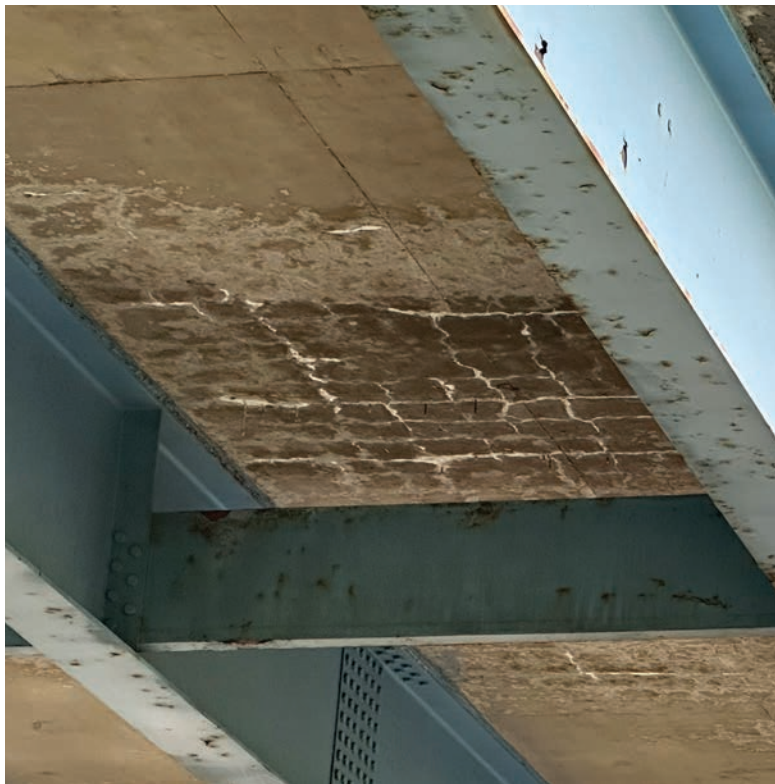
Deck cracking with efflorescence
