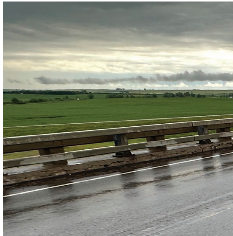
Spalling and cracking on bridge deck and curb sections
