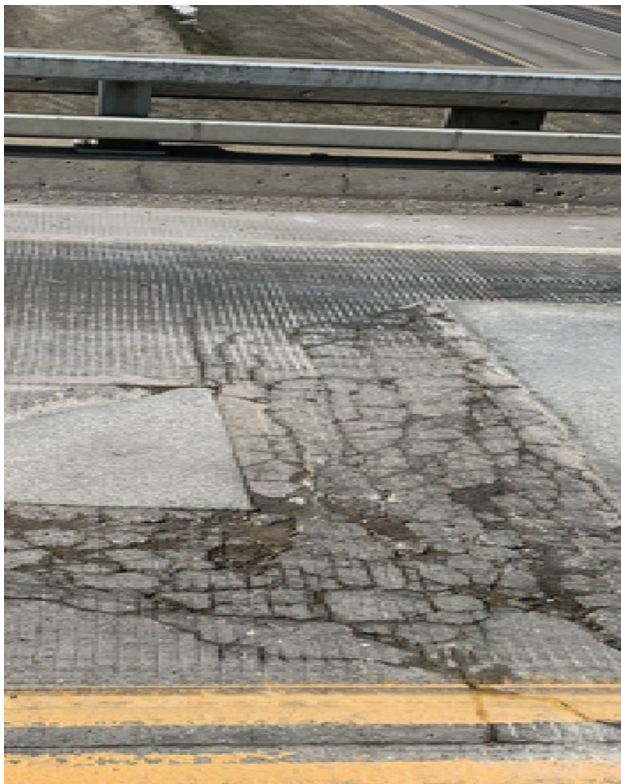
Deck cracking on roadway surface (photo taken prior to overlay)
