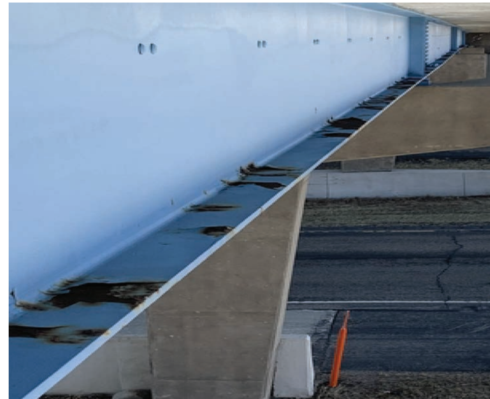
Steel corrosion and flaking paint
