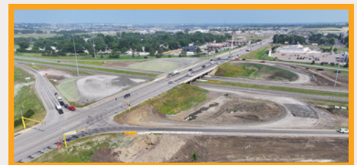
From the SE, looking at the two temporary loop ramps before paving
