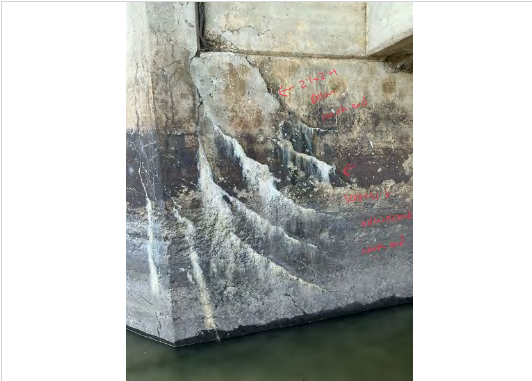
Facing East. U-Shaped Seepage and Efflorescence with Delam area to East Abutment North End.
