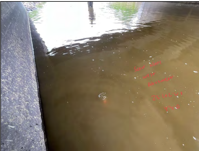
Facing North and Downward. Range Pole Submerged due to Scour along West Abutment.
