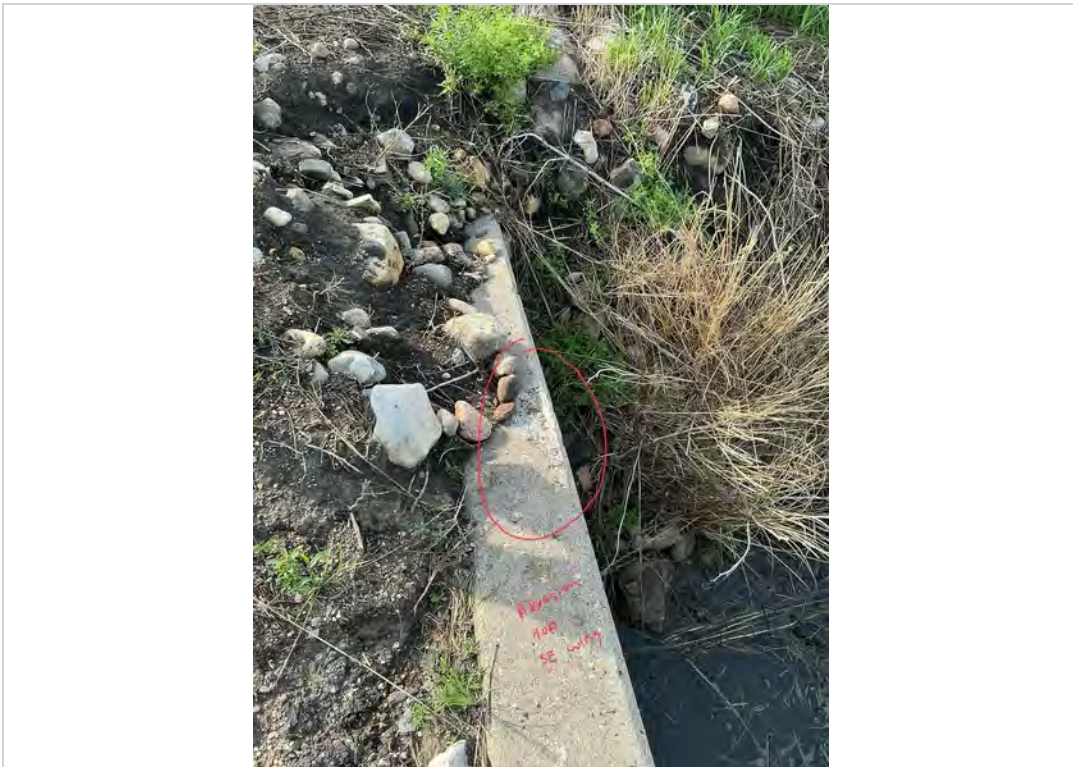
Facing SE and Downward. Abrasion along Top of SE Wing
