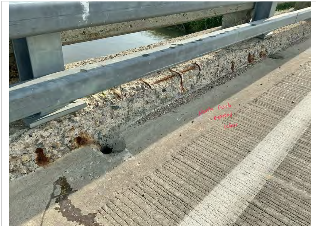
Facing NE. Abrasion with Exposed Rebar to North Curb.
