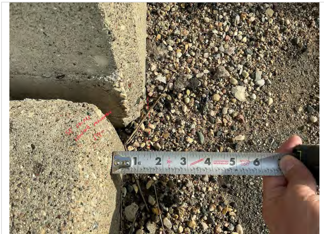
Facing North. SE Inward Movement at Top of Wing.
