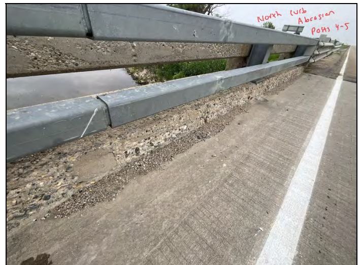
Facing NE. Moderate Abrasion along North Curb from Posts 4-5.
