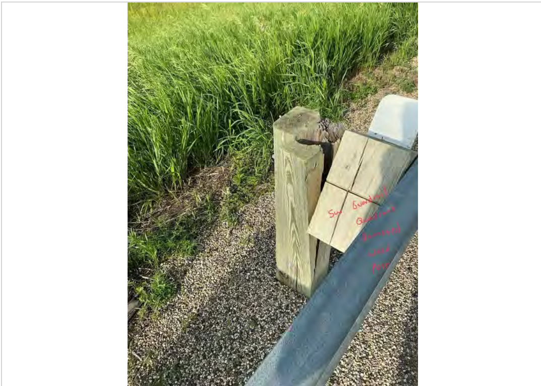
Facing SW. Cracked/Split Wood Post SW Guardrail Quadrant.
