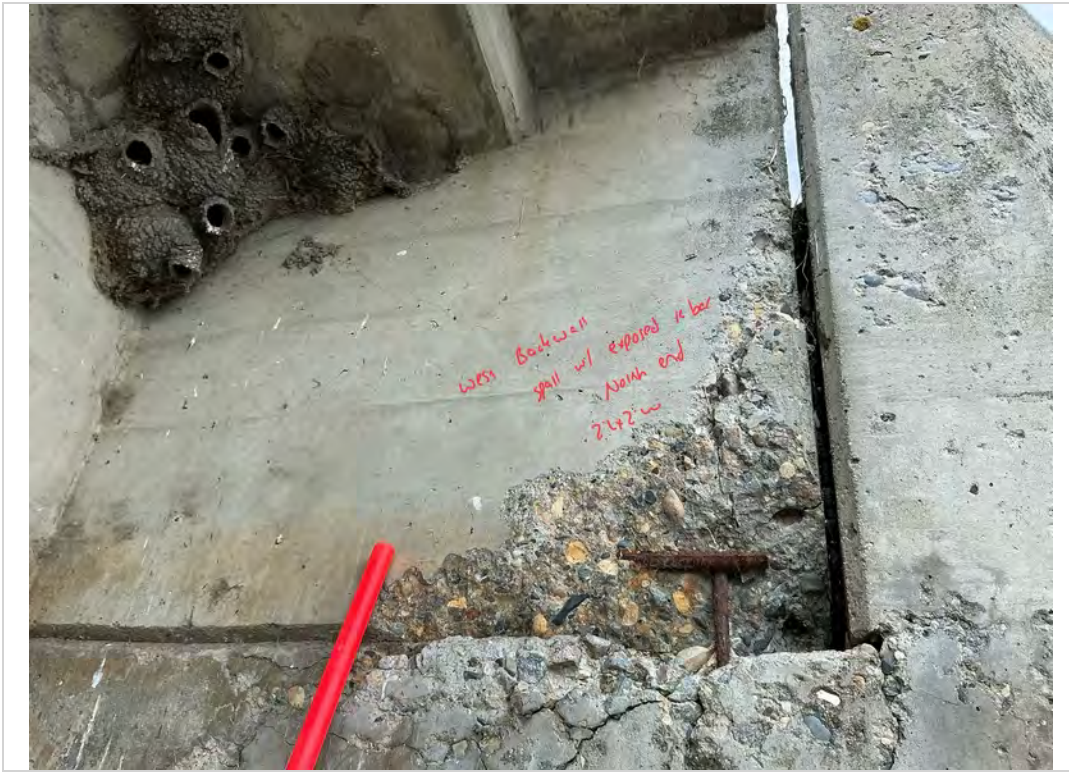
Facing West. Spalling with Exposed Rebar to West Backwall North End.
