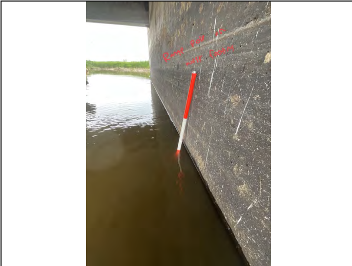
Facing South. Range Pole used to show Exposed Footing along Abutment.
