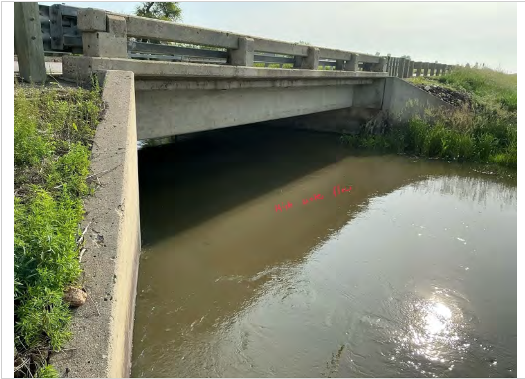
Facing NE. High Water Flow under structure.
