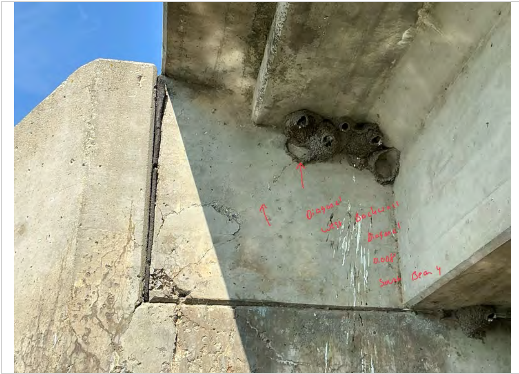
Facing West. Cracking to West Backwall South Beam 4.
