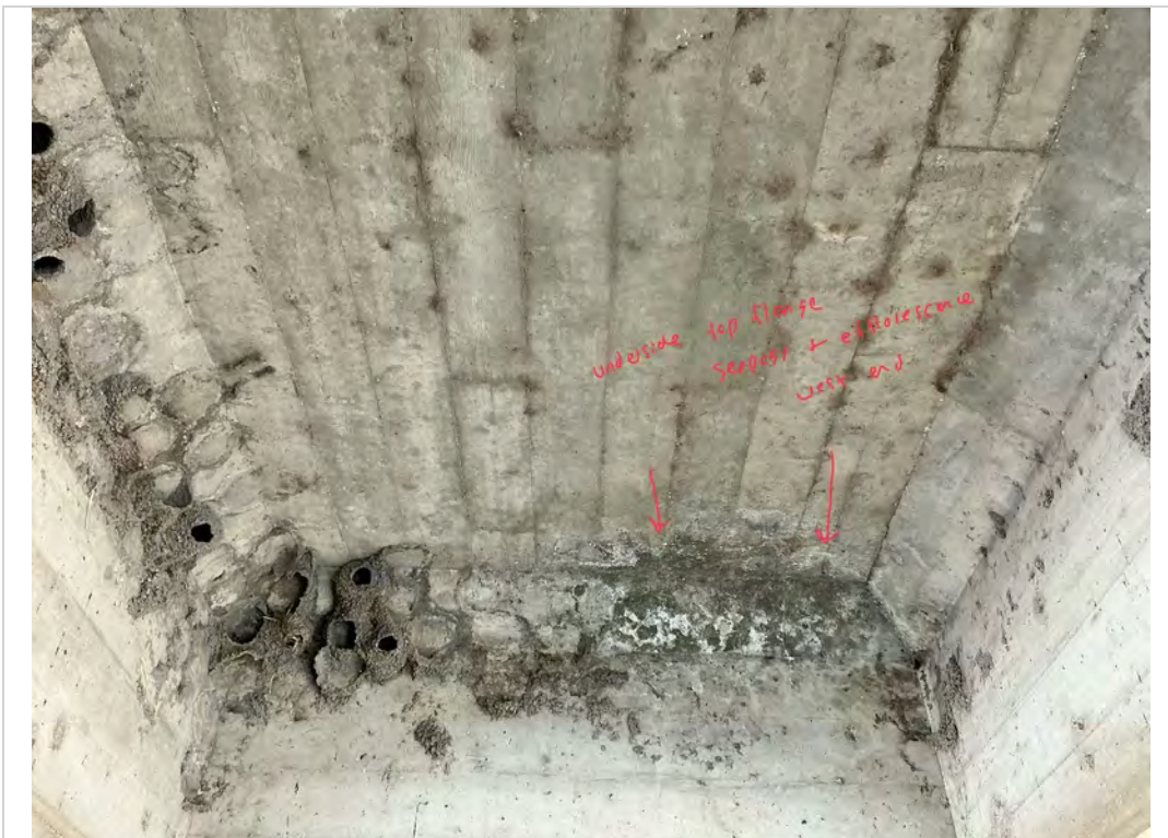
Facing West and Upwards. Seepage and Efflorescence to Underside Tee Beam West End.
