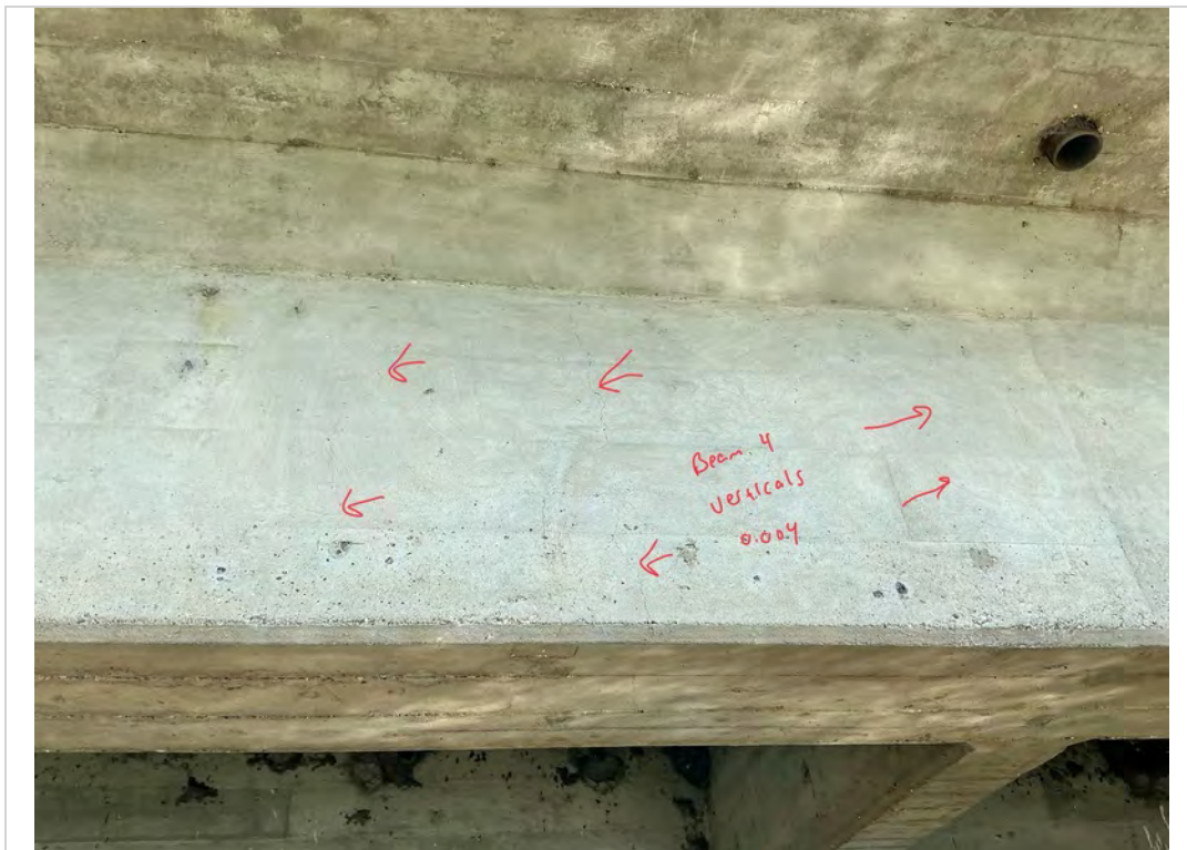
Facing North. Vertical cracks to Beam 4.
