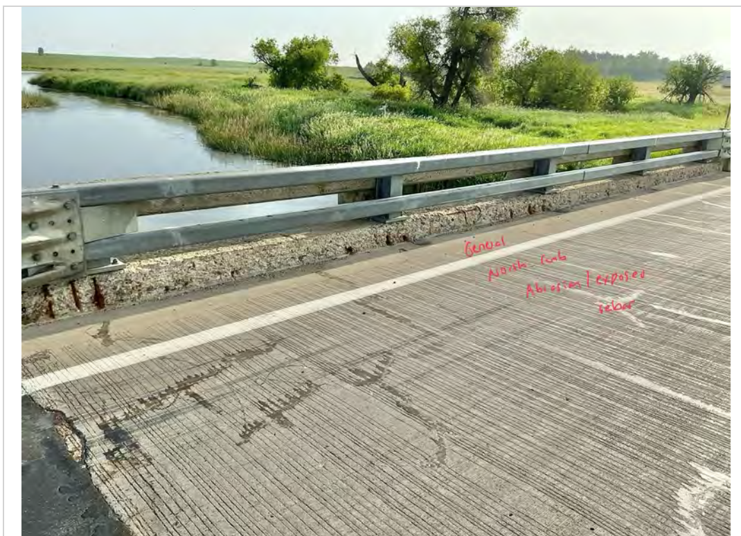
Facing NE. General of North Curb with Abrasion and Exposed rebar.
