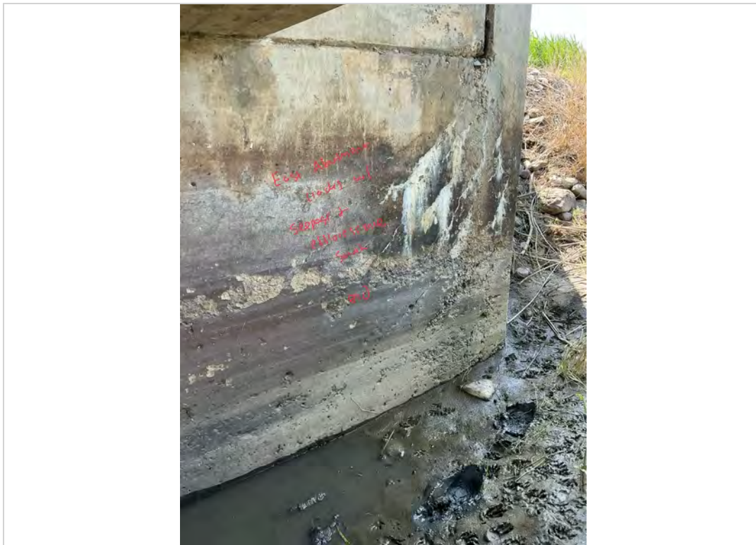
Facing SE. U-Shaped Cracking to East Abutment South end.
