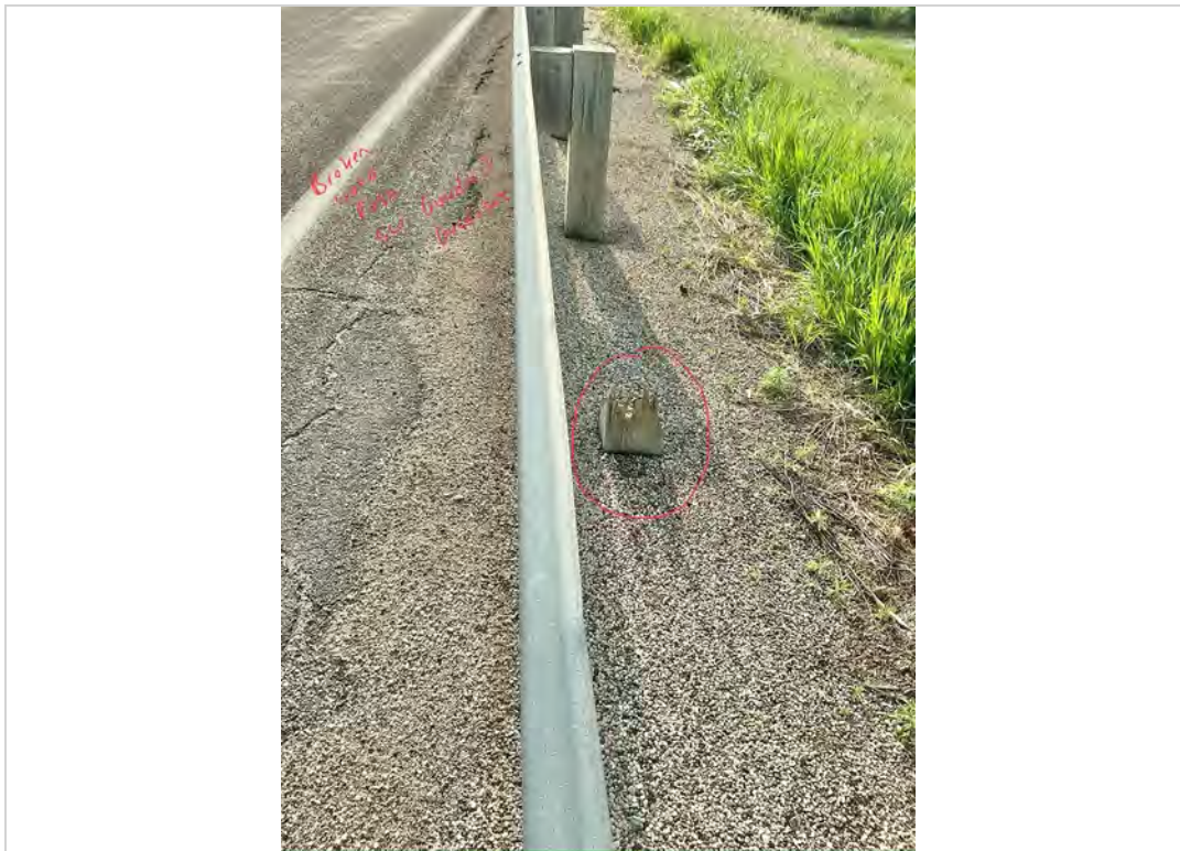
Facing East. Broken Wood Post SW Guardrail Quadrant.
