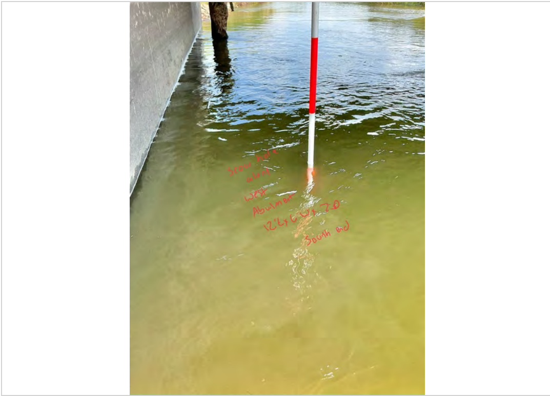
Facing North. Another View of the Scour Hole Depth along West Abutment near South End.
