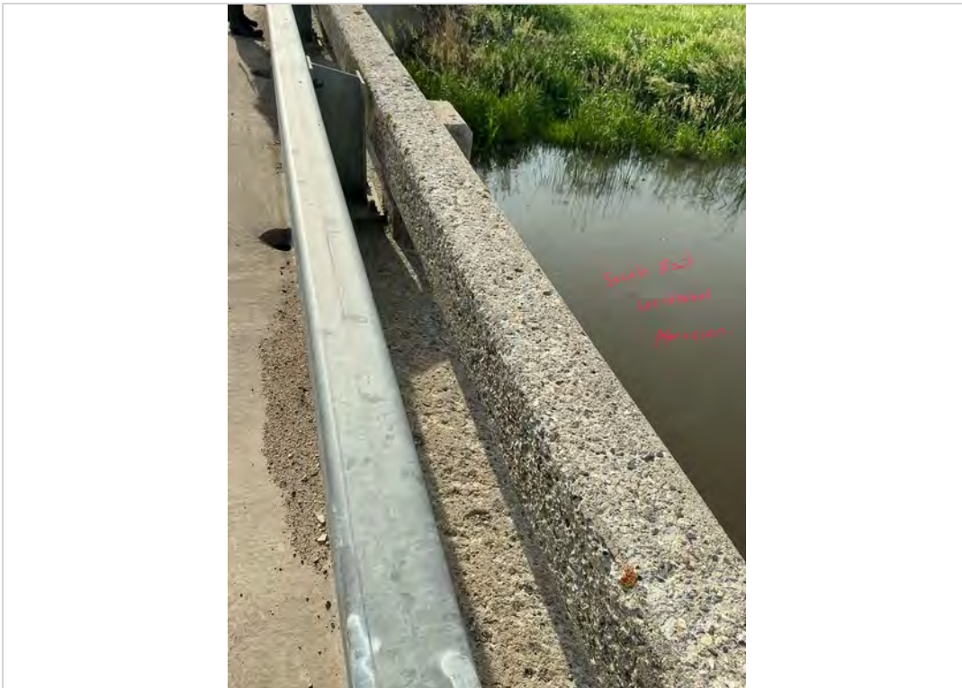
Facing East. South Railing Abrasion throughout.
