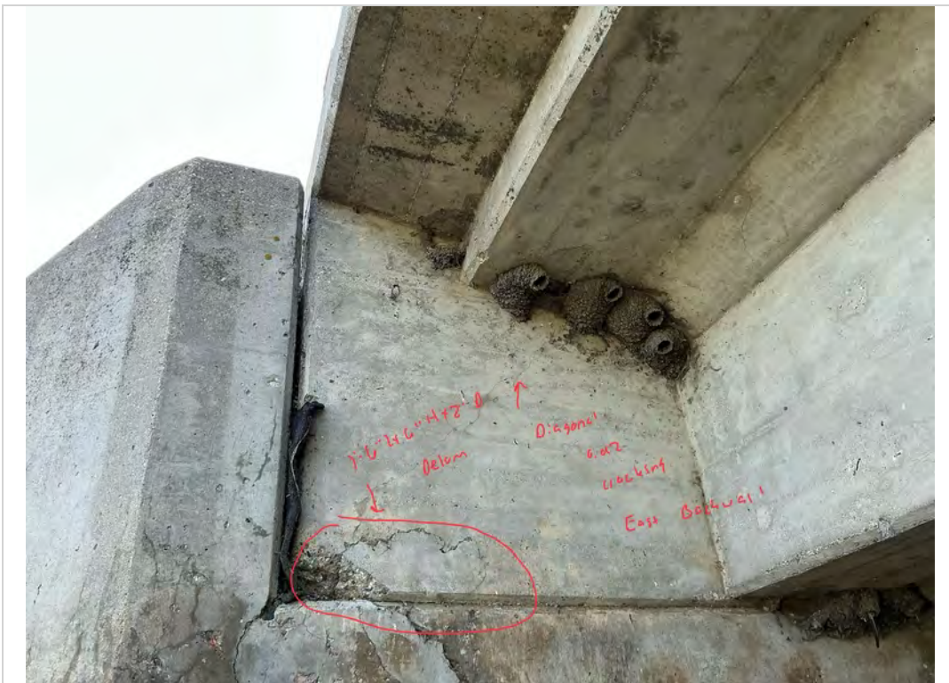
Facing East. Delam area and Diagonal Cracking to East Backwall North Beam 1.
