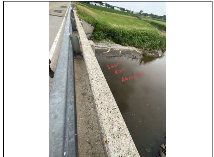
Facing East. Abrasion to South Railing.
