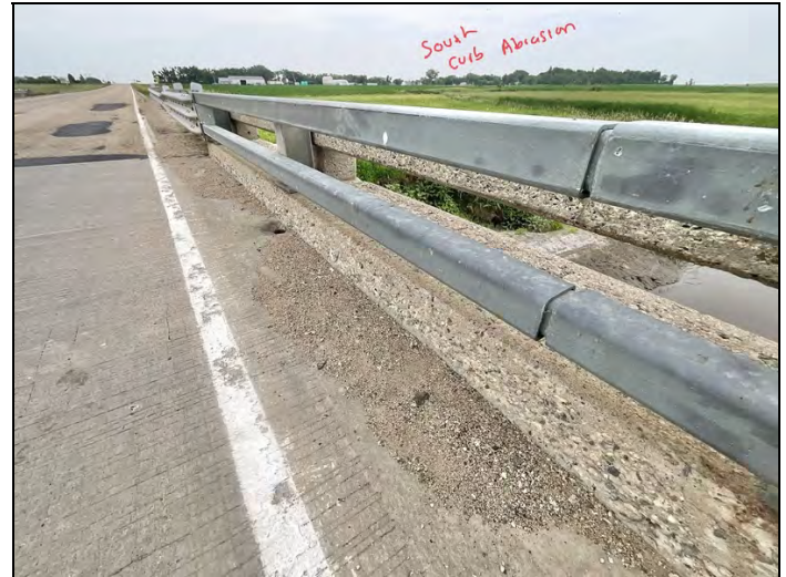
Facing East. Abrasion along South Curb.
