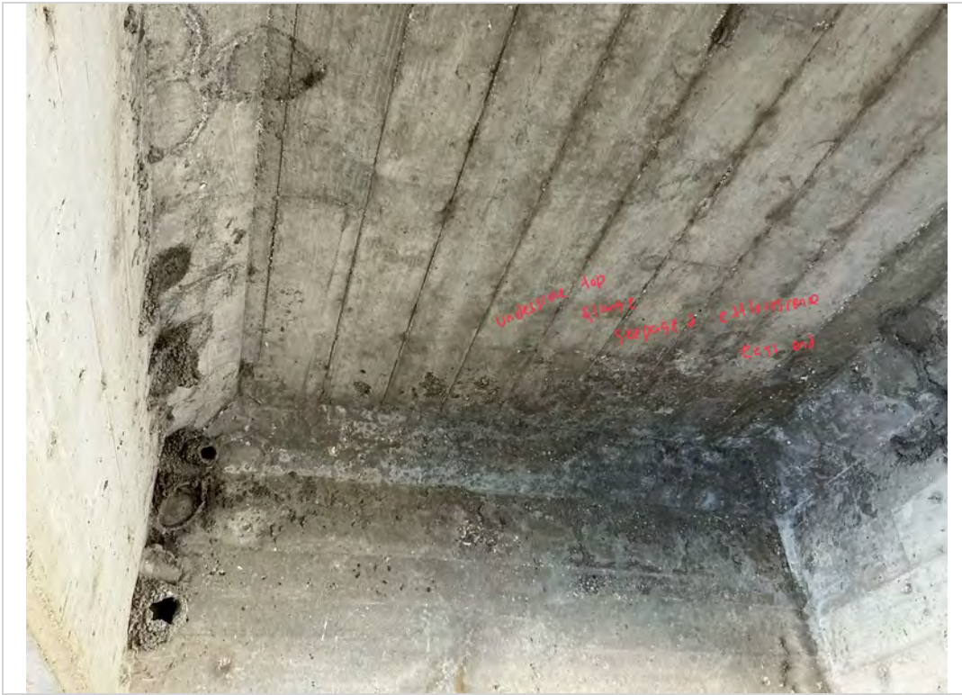
Facing East and Upwards. Underside Top Flange Seepage and Efflorescence East End.
