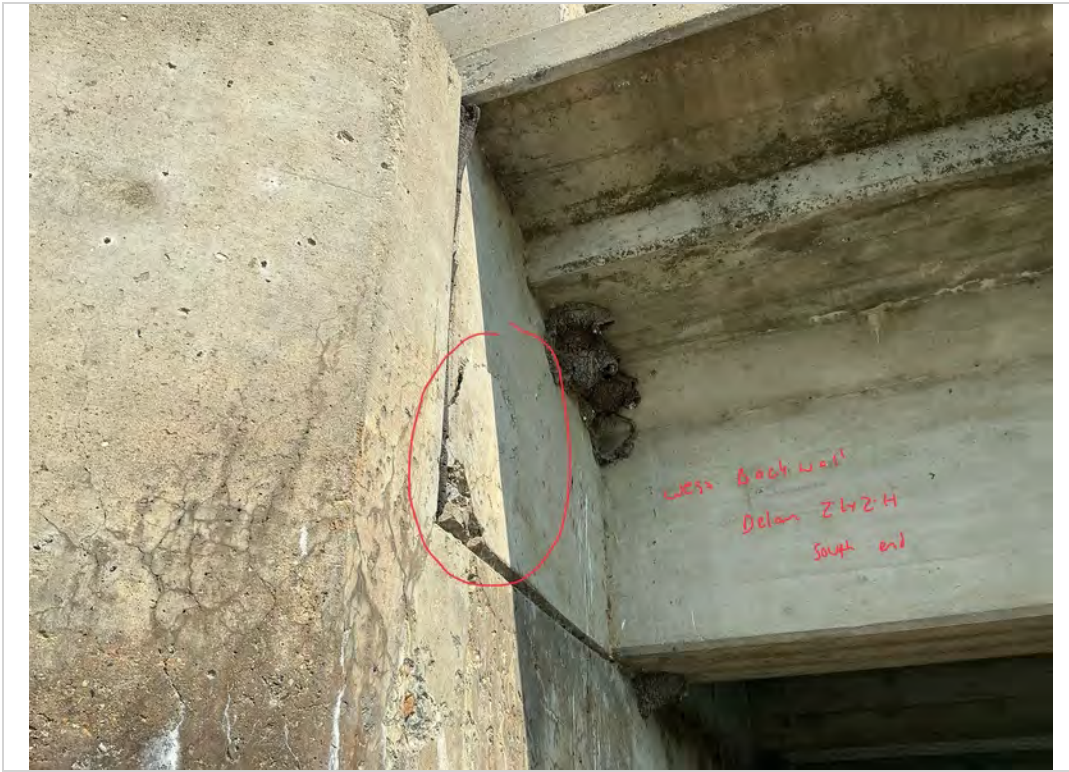
Facing North. Delam to West Backwall South End.
