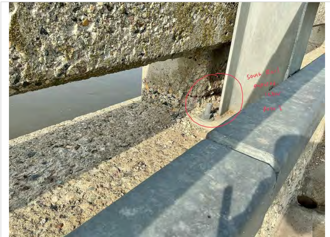
Facing SW. Exposed Rebar to South Railing Post 3.
