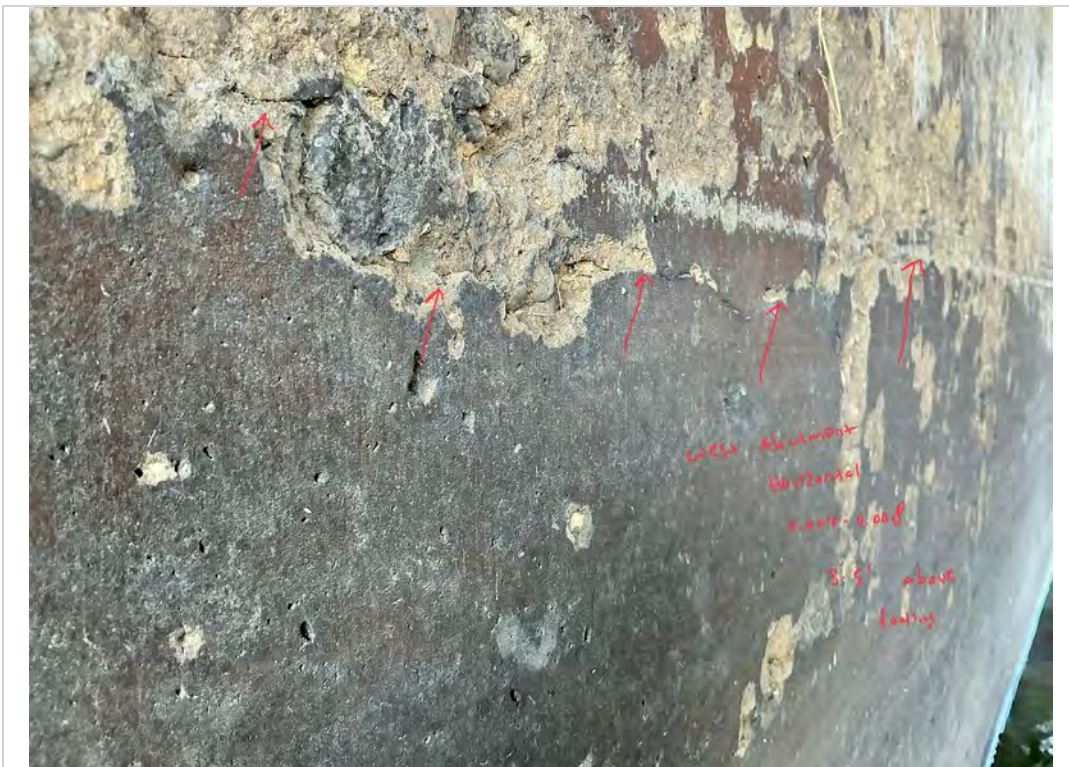
Facing NW. Minor Vertical and Horizontal Cracking to West Abutment.
