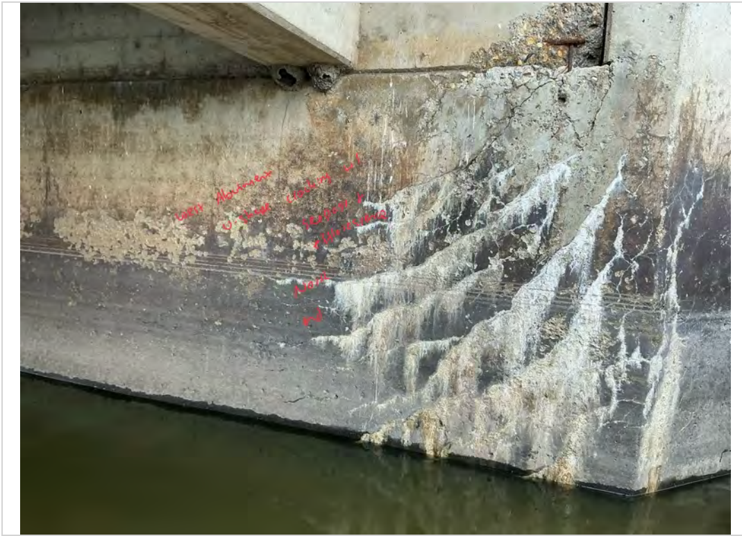
Facing West. U-Shaped Cracking with Seepage and efflorescence to West Abutment North end.
