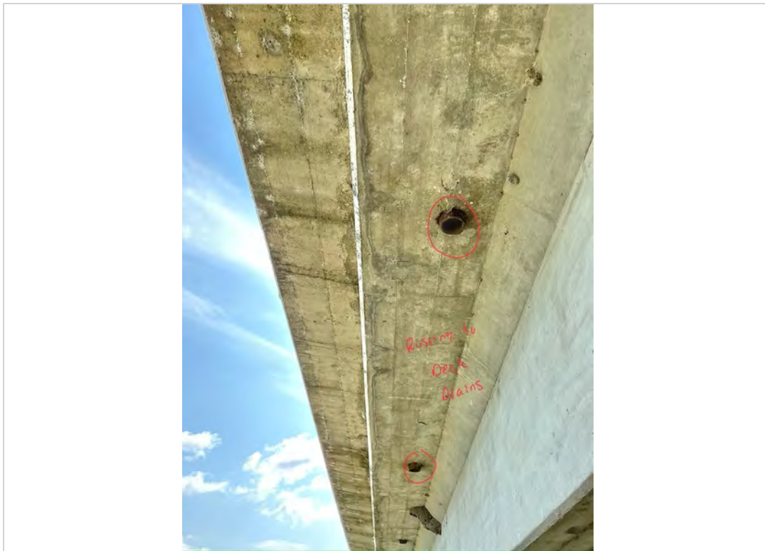
Facing East and Upwards. Rusting to Deck Drains.
