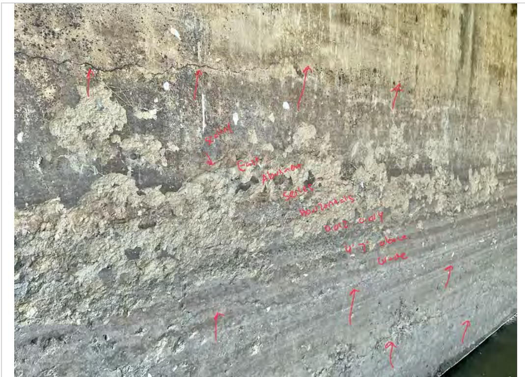
Facing SE. Some Minor Scaling with Series Horizontal Cracking to East Abutment.
