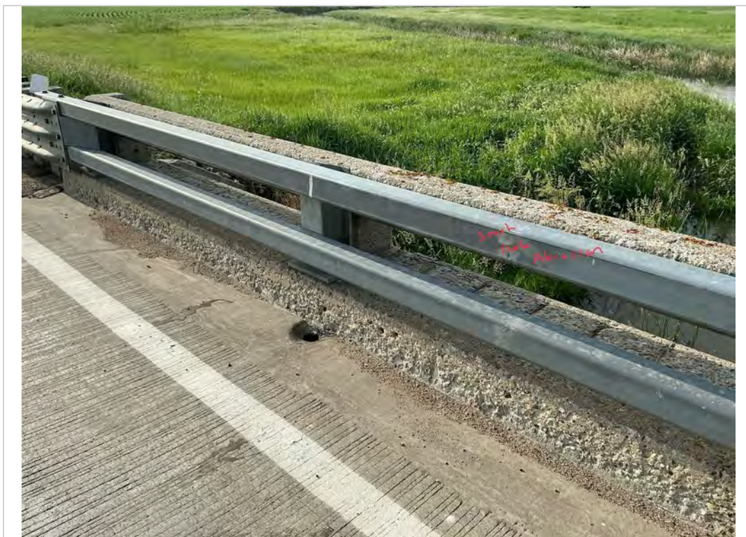
Facing SE. Continued Abrasion to South Curb and Railing.
