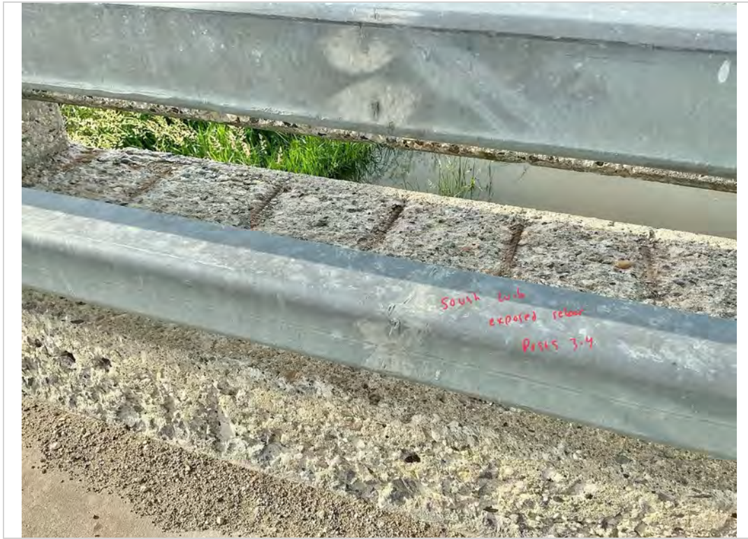
Facing South. Exposed Rebar to Top of South Curb.
