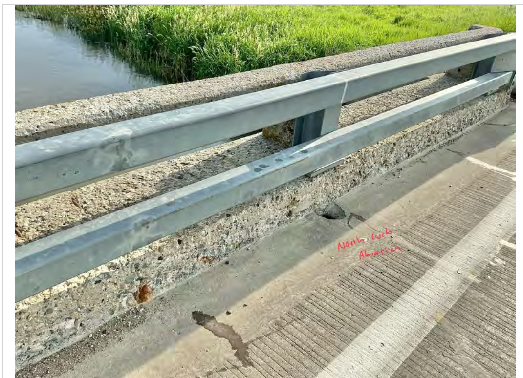
Facing NE. Abrasion to North Curb East End
