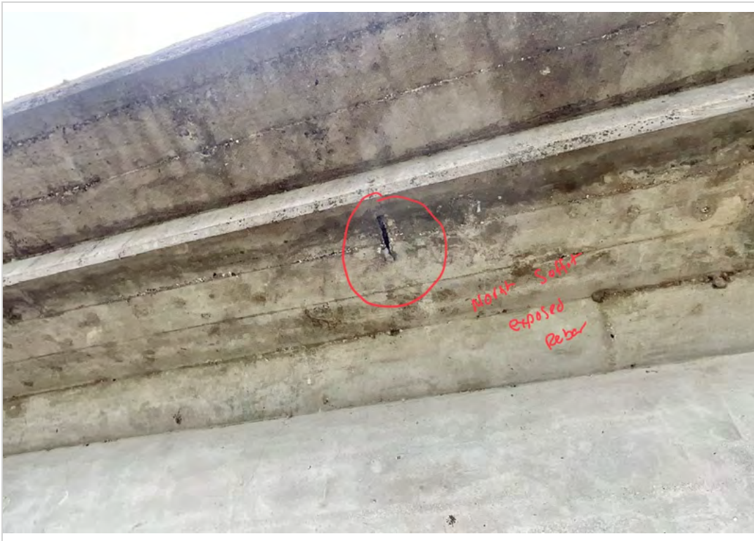
Facing South and Upwards. Exposed rebar to North Soffit of Top Flange Deck.
