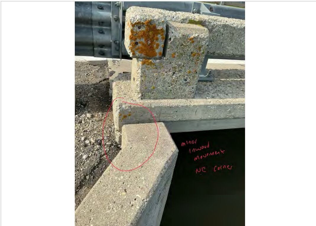
Facing South. Inward Movement at NE Corner.
