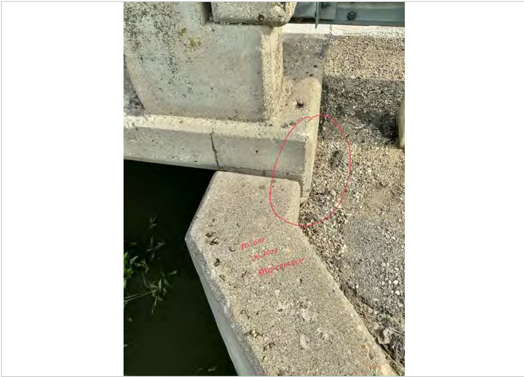
Facing North. Inward Movement at Top, SE Corner. Typical all Corners.
