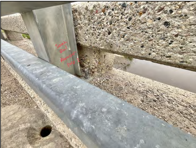
Facing SE. Moderate Abrasion to South Rail Post 3.
