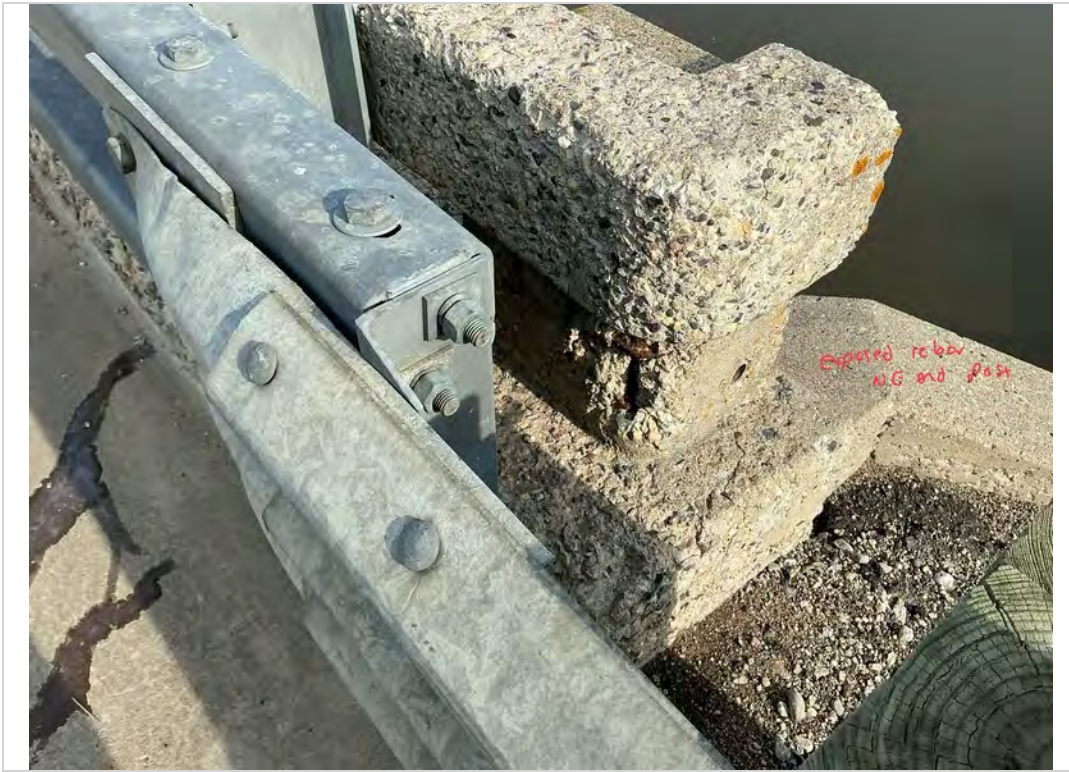
Facing NW. Exposed Rebar to NE End Post.
