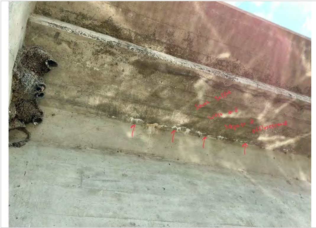
Facing North and Upwards. South Soffit with Seepage and Efflorescence.
