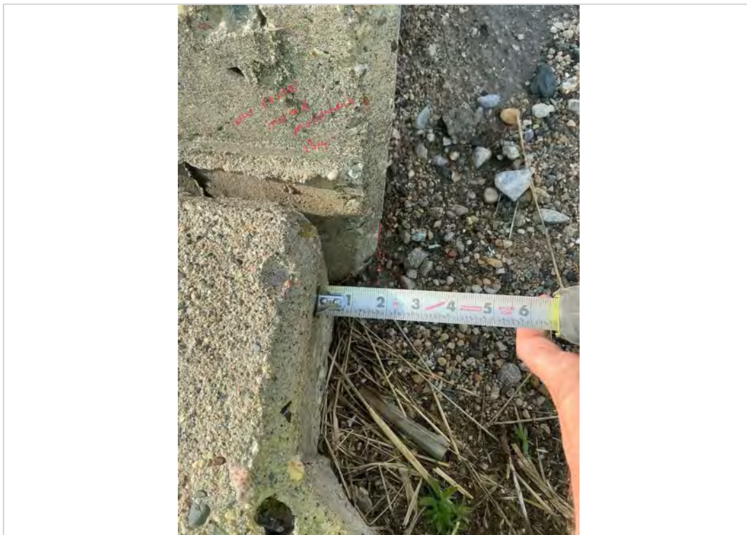
Facing South and Downward. Inward Movement of NW Corner of Structure.
