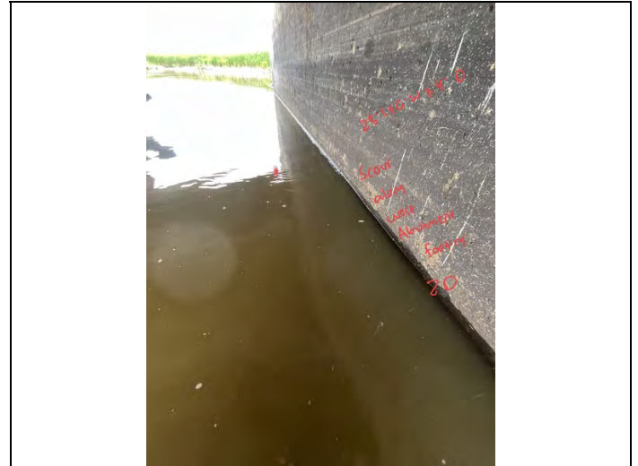
Facing South. Range Pole used to determine area of Scour along West Abutment.
