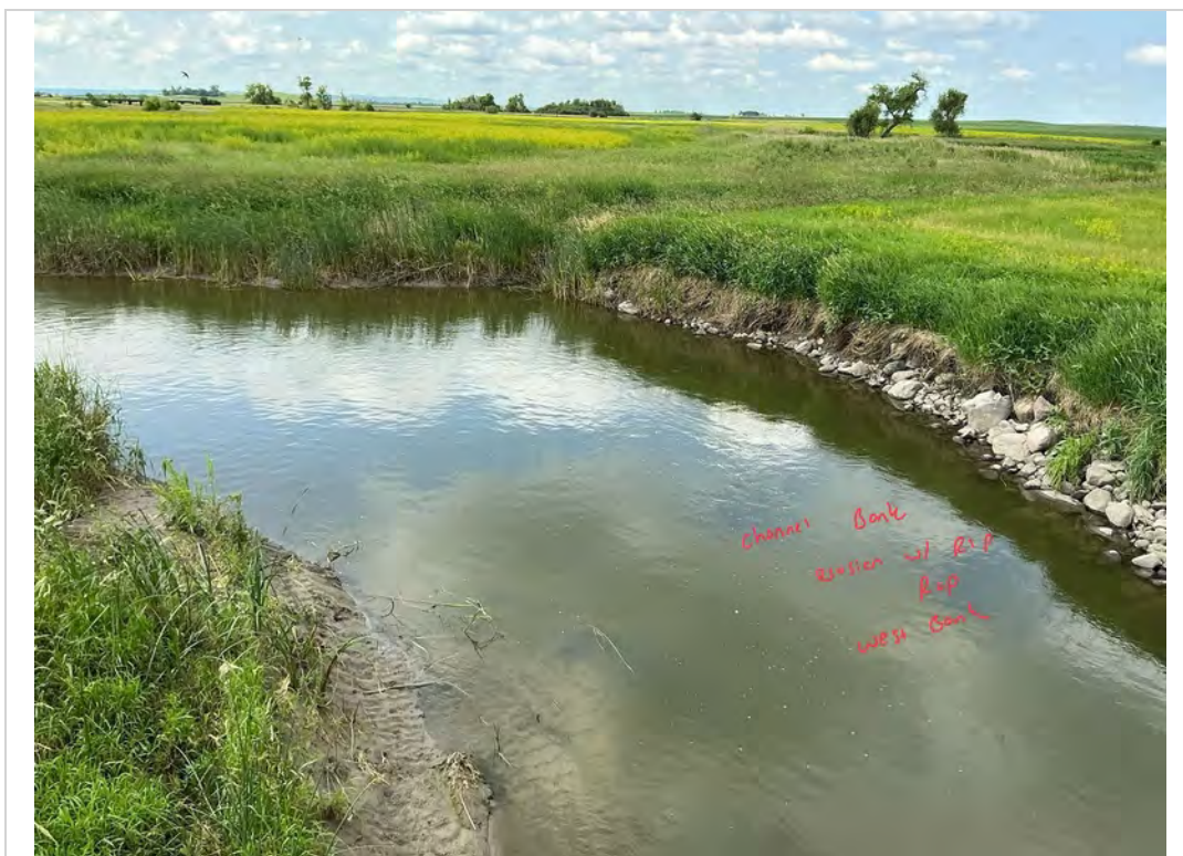
Facing SW. Channel Bank Erosion along West Side of Bank South of Structure.
