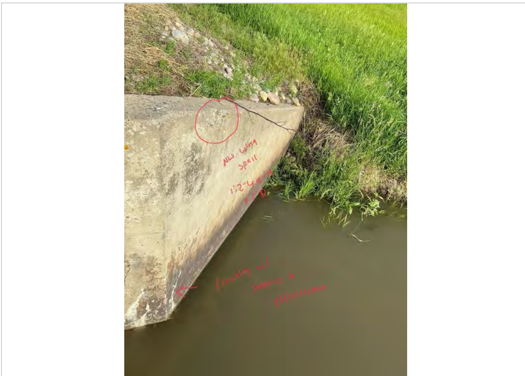
Facing West. Spall along Top with Cracking, Seepage, Efflorescence to NW Wing.
