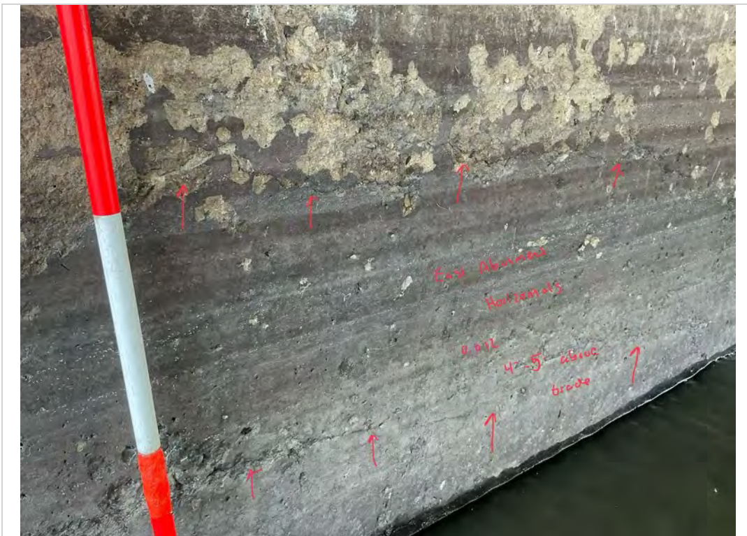
Facing SE. Continued Series of Horizontal Cracking to East Abutment
