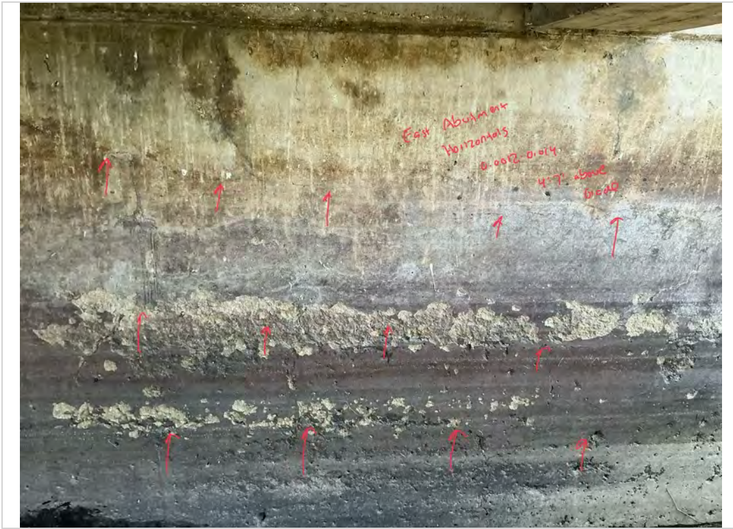
Facing East. Series of Horizontal Cracking to East Abutment.
