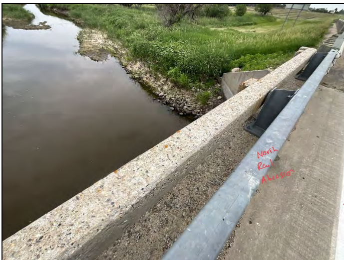
Facing NE. Abrasion along North Railing.
