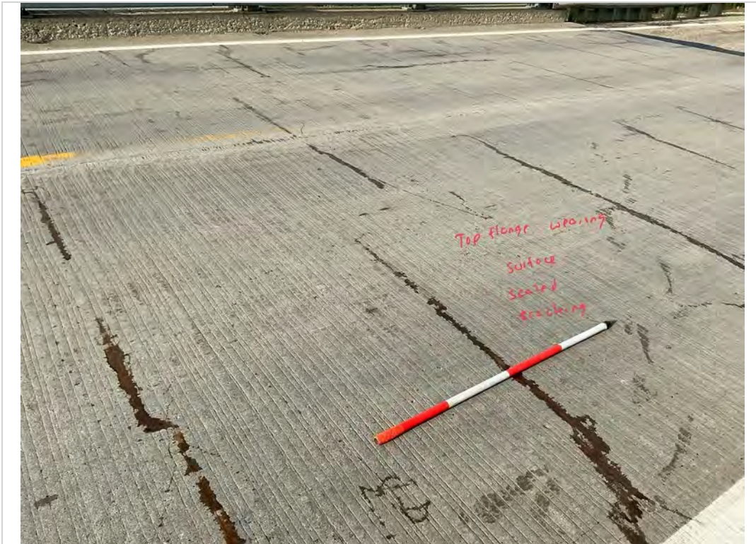
Facing South. Sealed Transverse Cracking to Top Flange Deck Wearing Surface.
