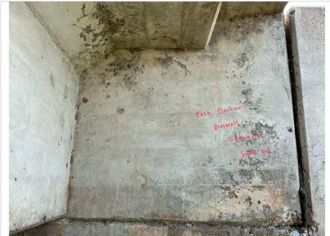
Facing East. Diagonal Cracking to East Backwall South End.
