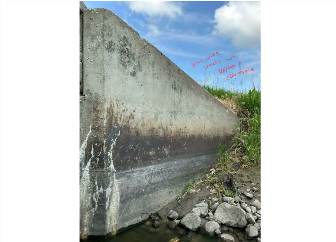
Facing West. NW Wing with Cracking, Seepage, and Efflorescence.
