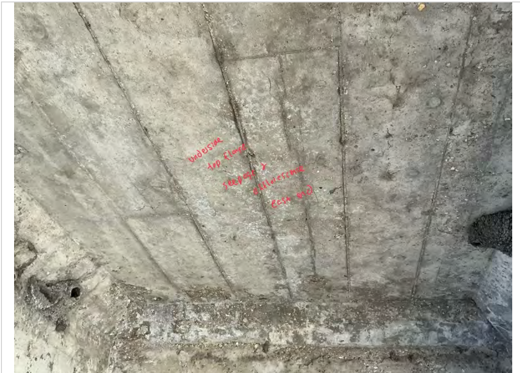
Facing East and Upwards. Underside Top Flange Deck with seepage and efflorescence East End.
