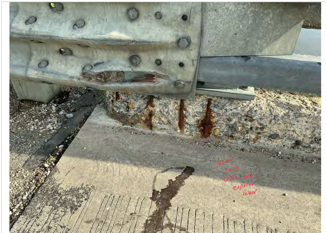
Facing North. Exposed Rebar to North Curb West End.
