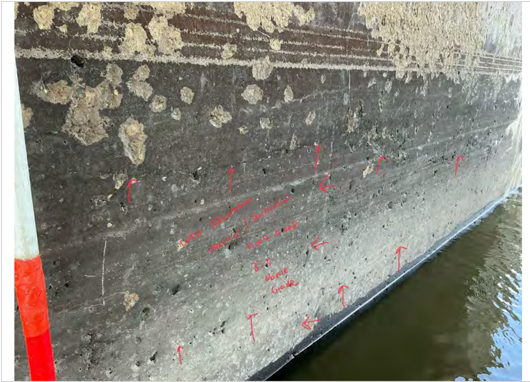
Facing NW. Vertical and Horizontal Cracking to West Abutment near North End.
