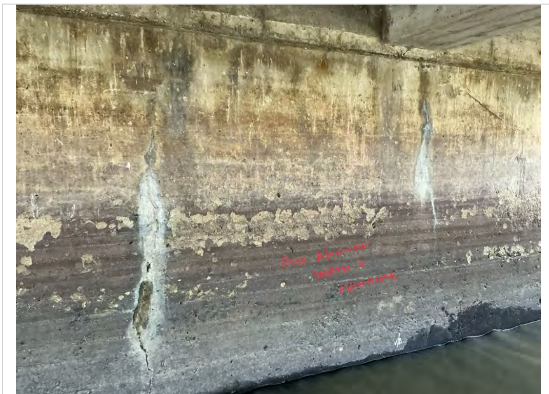
Facing East. Vertical Cracks with Seepage and Efflorescence to East Abutment.
