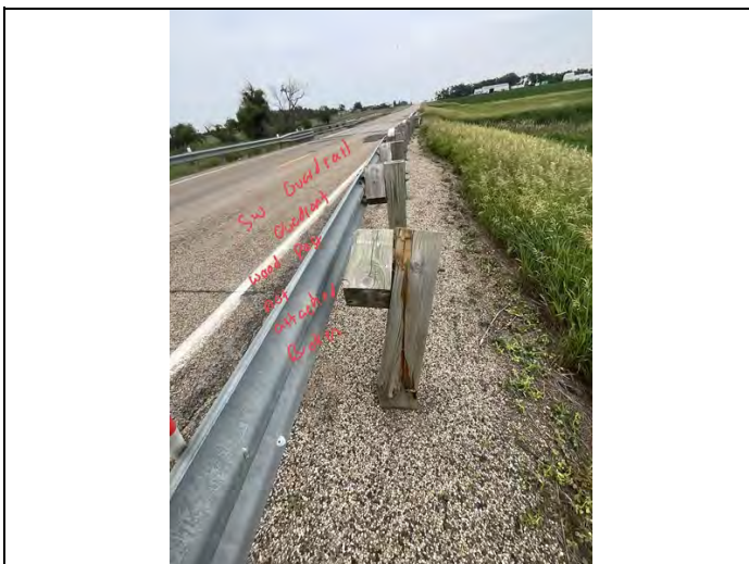
Facing East. Cracked and Broken Wood Post not attached to W-Beam SW Quadrant.
