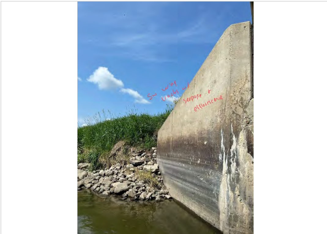
Facing West. Seepage and Efflorescence to SW Wing.
