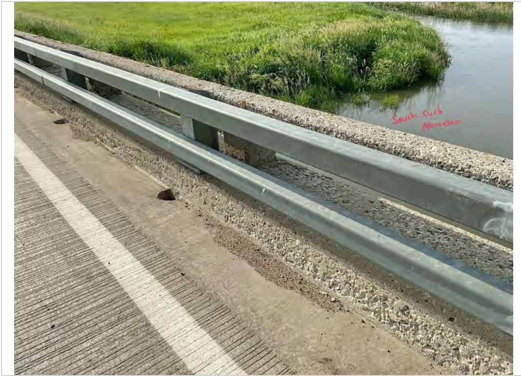
Facing SW. South Curb Abrasion.
