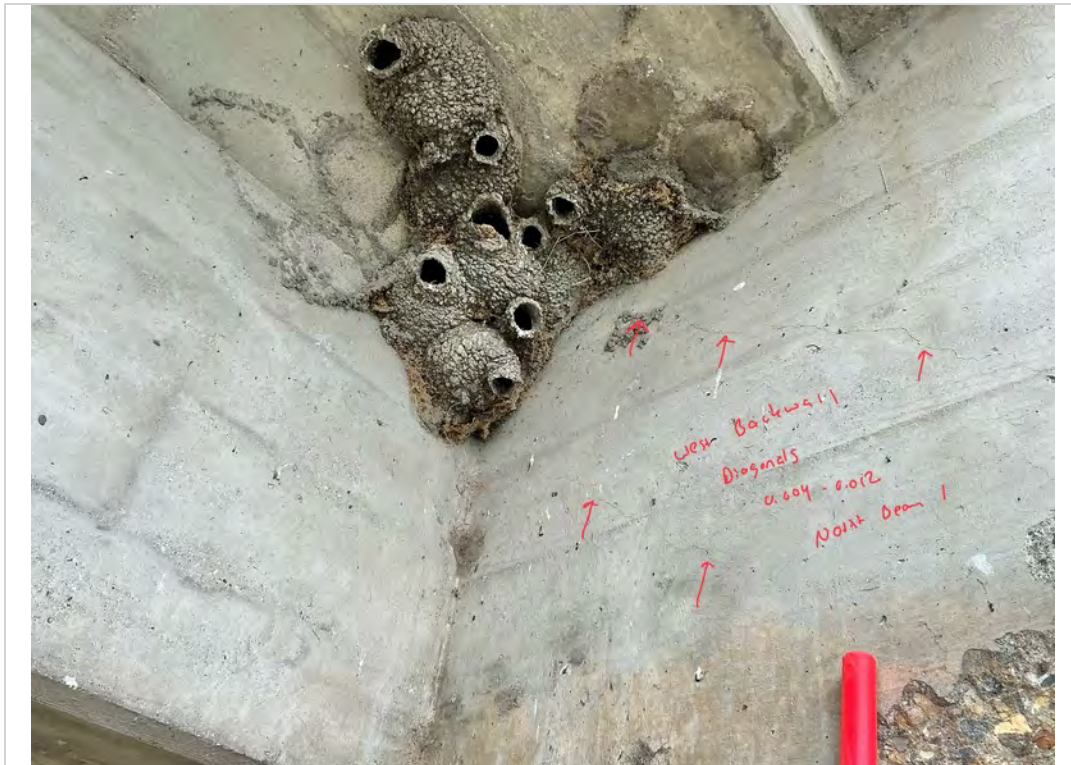
Facing SW and Upwards. Diagonal Cracks to West Backwall North Beam 1.
