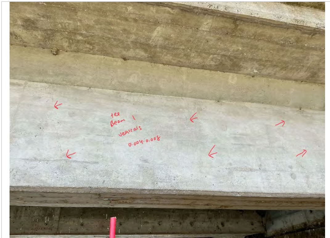
Facing South. Minor Vertical cracks to Beam 1.
