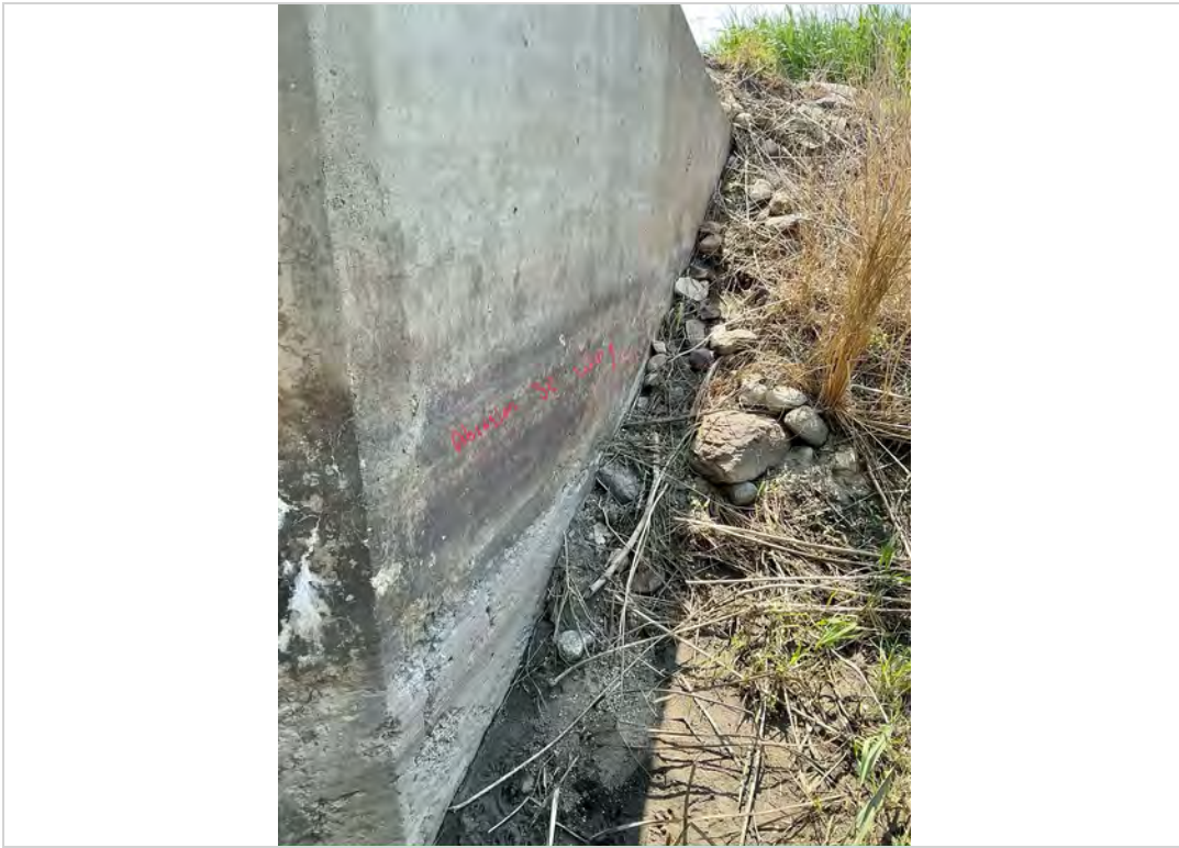
Facing East. Abrasion along Face of SE Wing.
