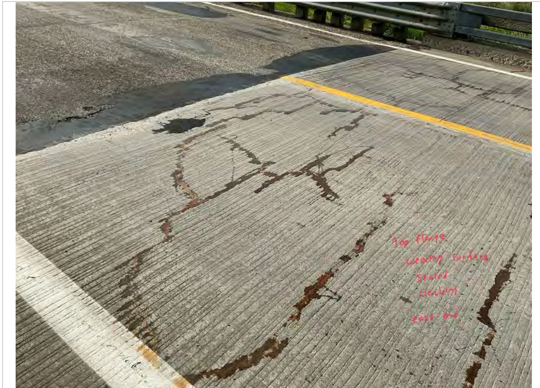
Facing SE. Sealed Cracking to Top Flange Deck Wearing Surface East End.
