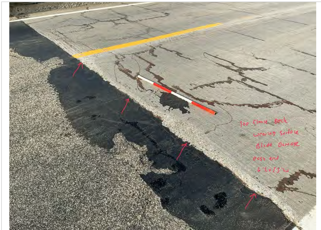
Facing SW. Blade Damage to East End of Top Flange Deck Wearing Surface.
