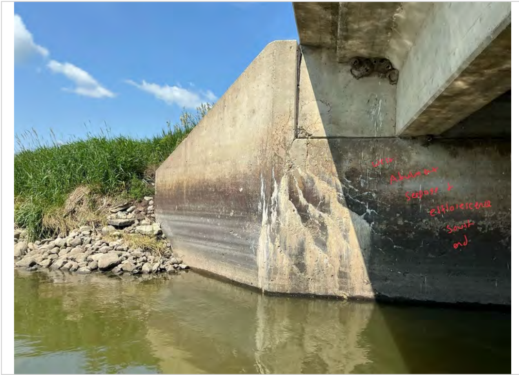
Facing West. U-Shaped Cracking with Seepage and Efflorescence to West Abutment South End.
