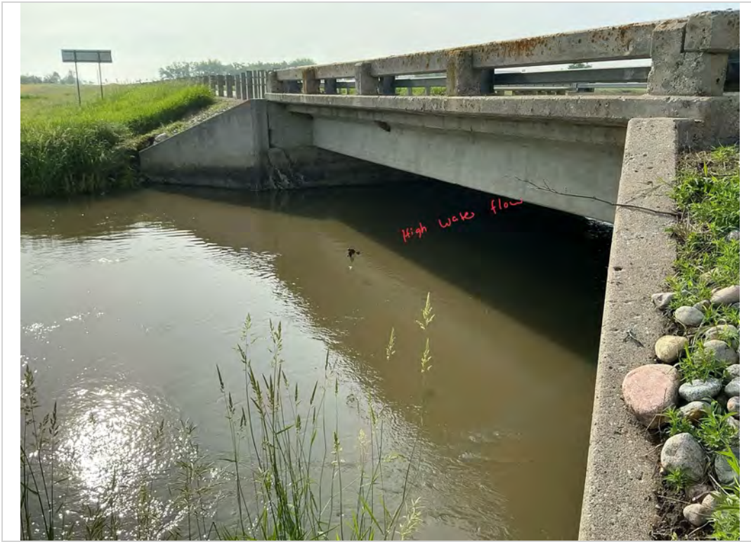
Facing SE. High Water Flow under structure.
