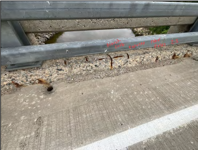
Facing North. Exposed Rebar to North Curb in-between Posts 2 and 3.
