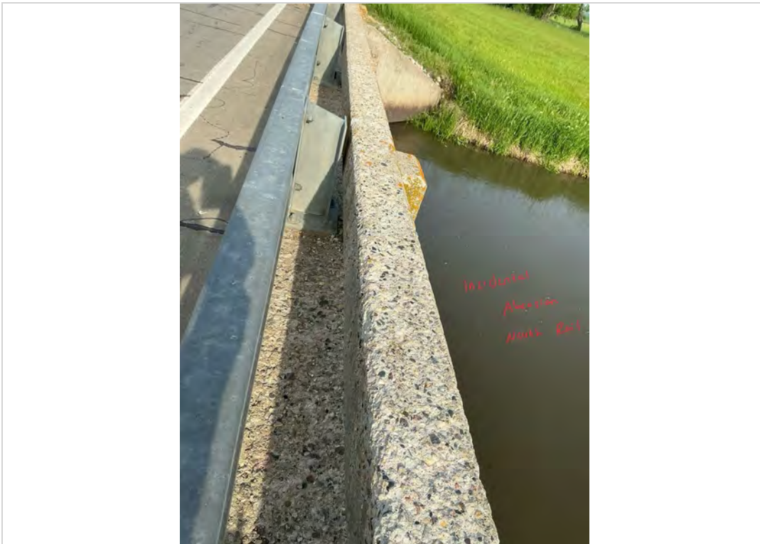
Facing West. Abrasion along North Railing.
