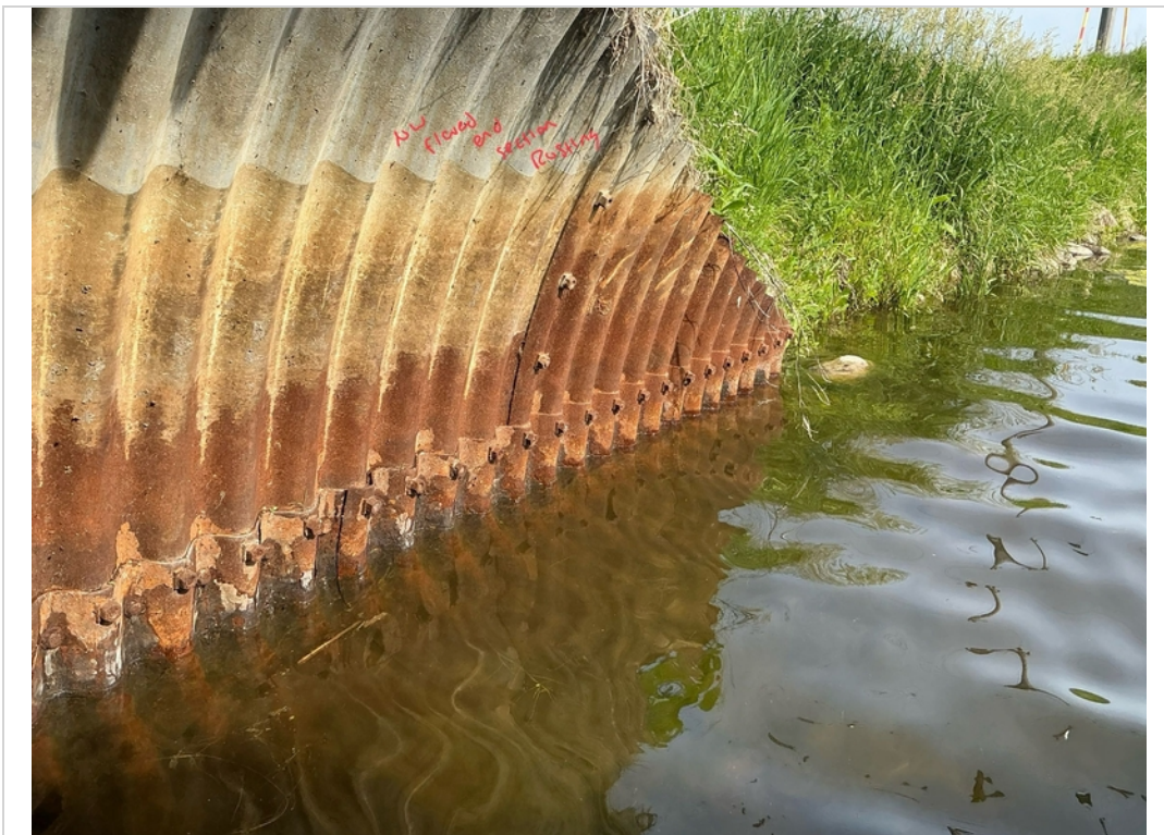
Facing North. Rusting to NW Flared End Section. Typical
