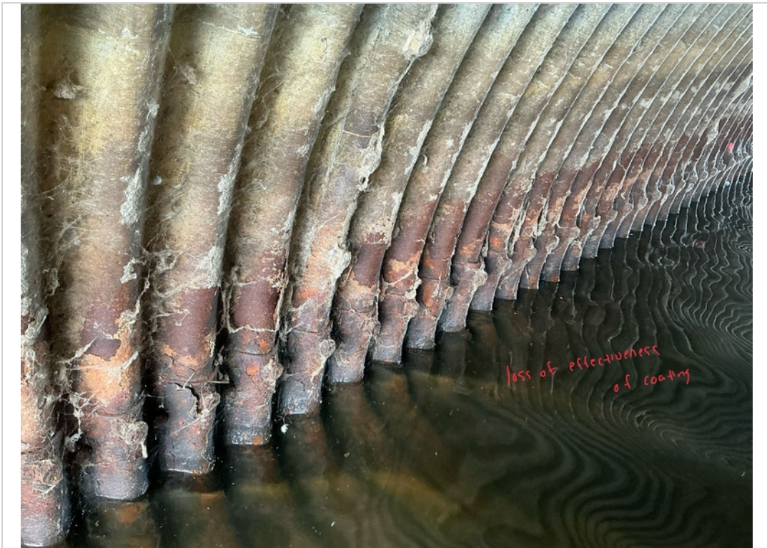
Facing NW. Loss of Effectiveness of coating
