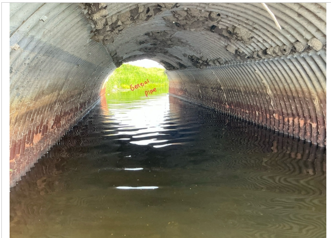
Facing North. General of Pipe.
