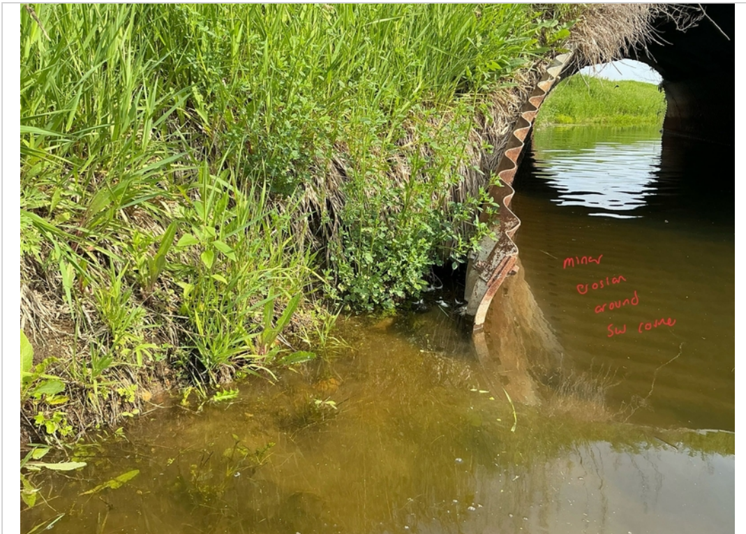
Facing North. Minor Erosion around SW Flared end Section. Typical all corners.
