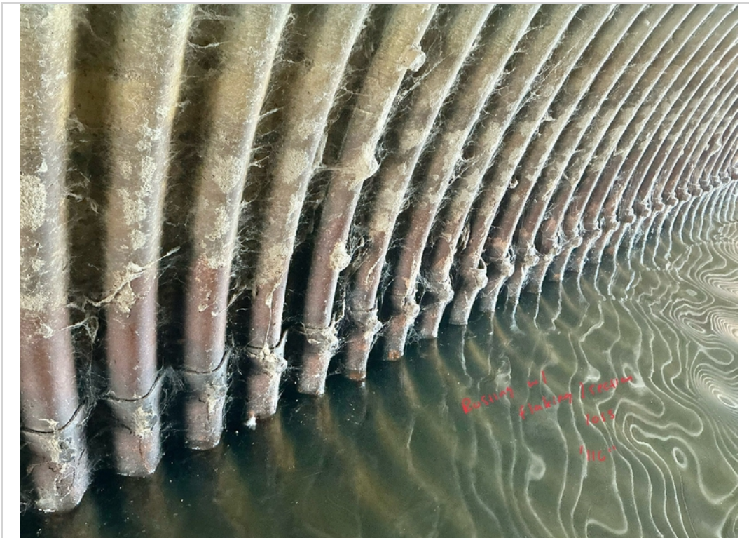
Facing NW. Rusting with Flaking and Section Loss to Lower Portion of Pipe along Connection Seam.
