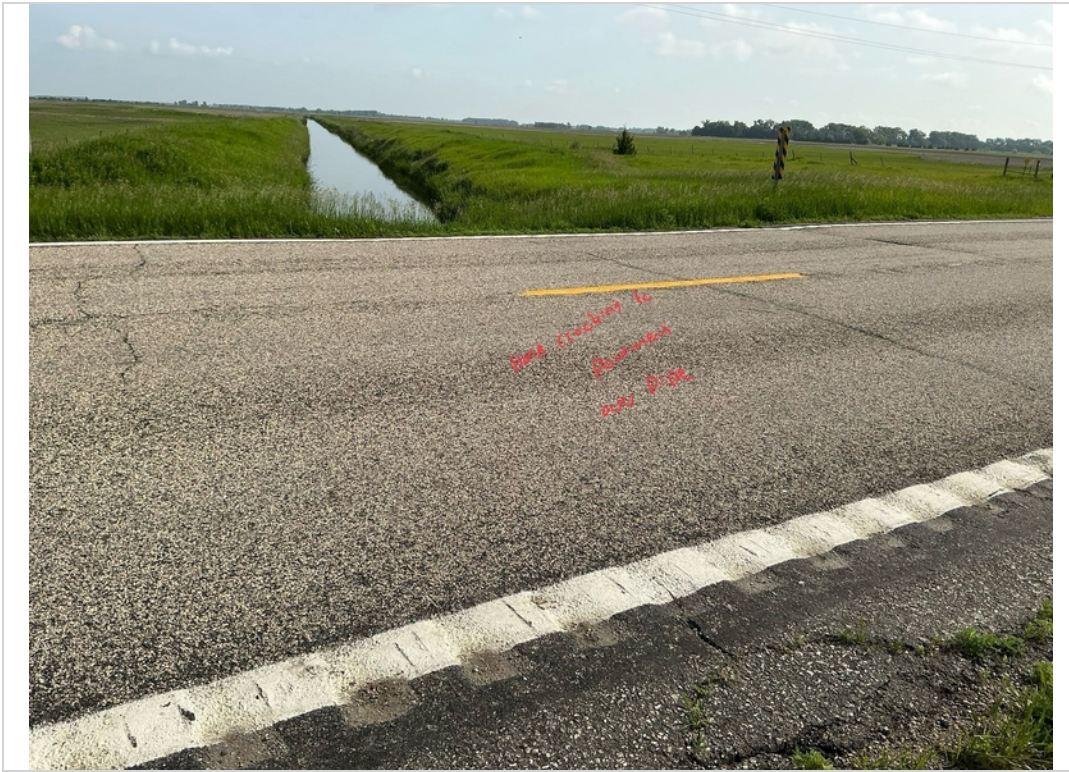
Facing North. Cracking to HMA Pavement over Pipe.
