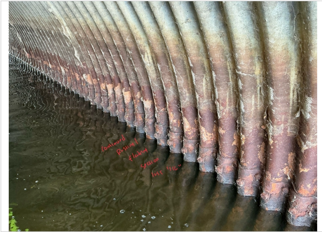
Facing NE. Moderate Rusting with Flaking and Section Loss to Pipe.
