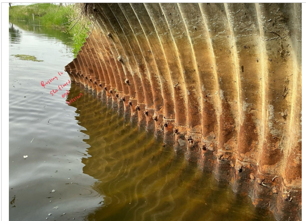
Facing SW. Rusting to South Flared End Section. Typical all Corners.
