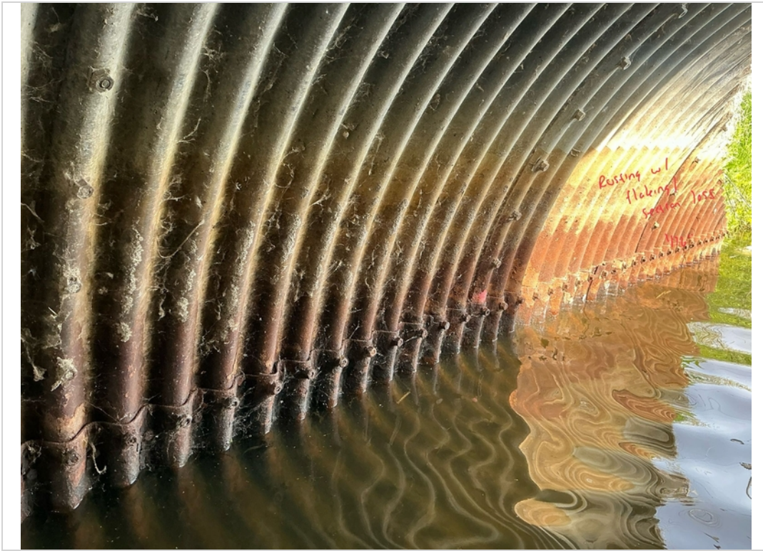
Facing NW. Rusting with Flaking and Section Loss to Pipe Sides.
