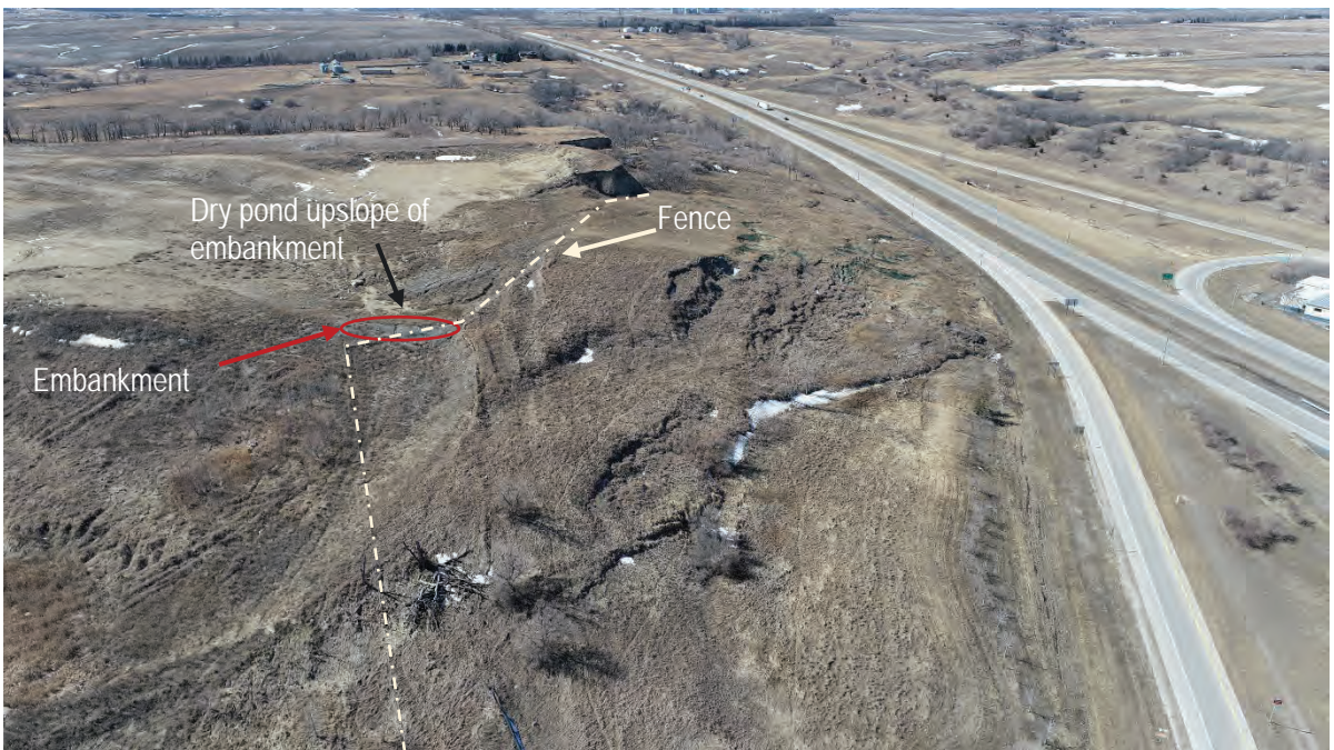
Exhibit 3-4: Site Reconnaissance Photo 4 - View of the slide mass with location of embankment and dry pond, facing west.
