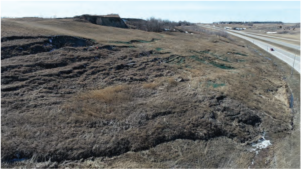
Exhibit 3-3: Site Reconnaissance Photo 3 - View of part of the slide mass with the overriding toe feature, facing west. Note the person in the orange vest in the upper left for scale.
