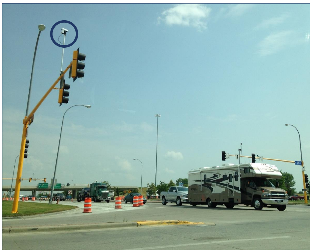
Figure 26: Video Detection System on US 2
