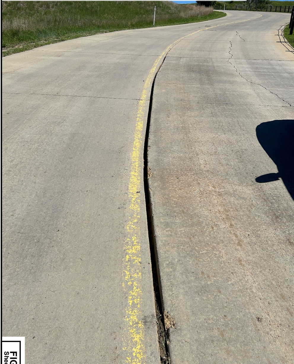
View northeast showing pavement distress at site Feature 6. Photograph taken June 11, 2024.
