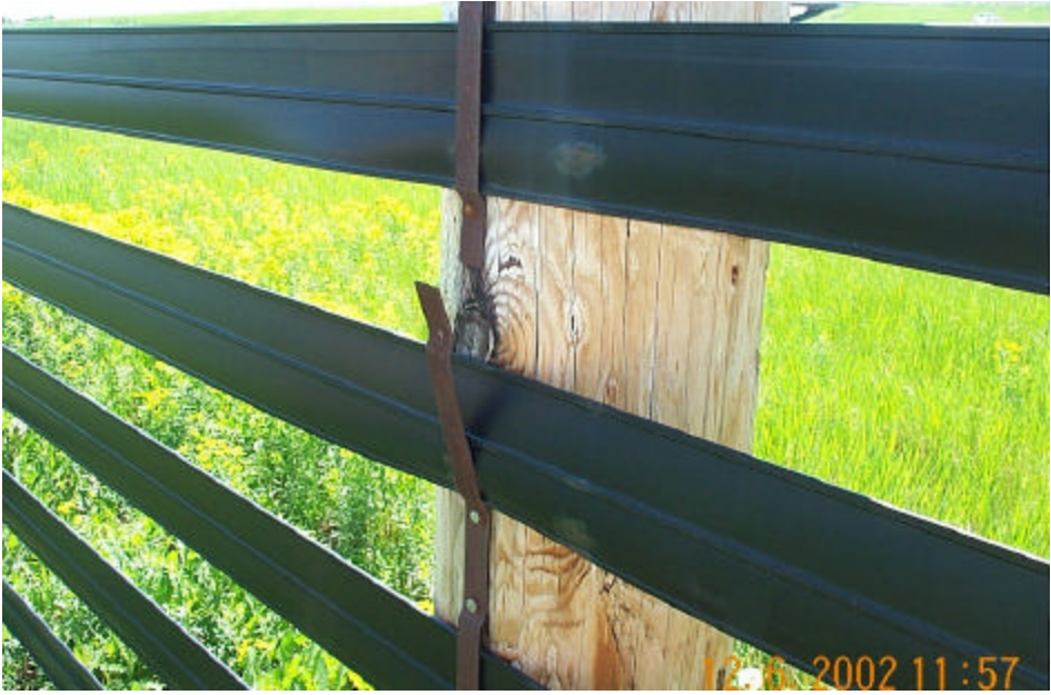
Photo 4 - Bracket that has become loose.
