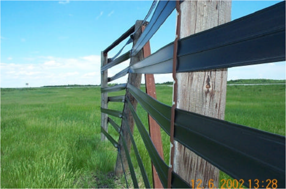
Photo 5 - A tilted fence post at Site 4.
