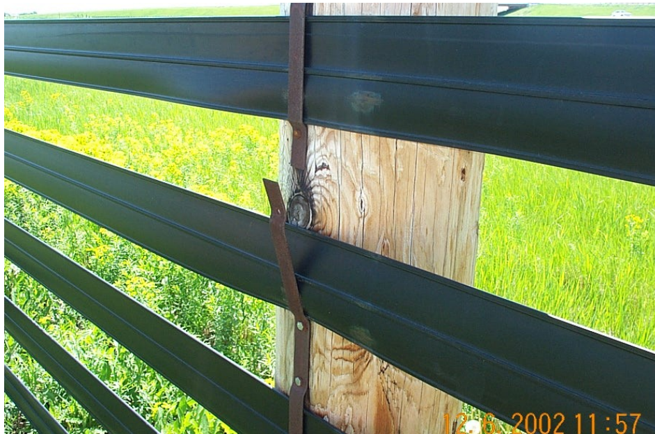
Photo 4 - Bracket that has become loose.
