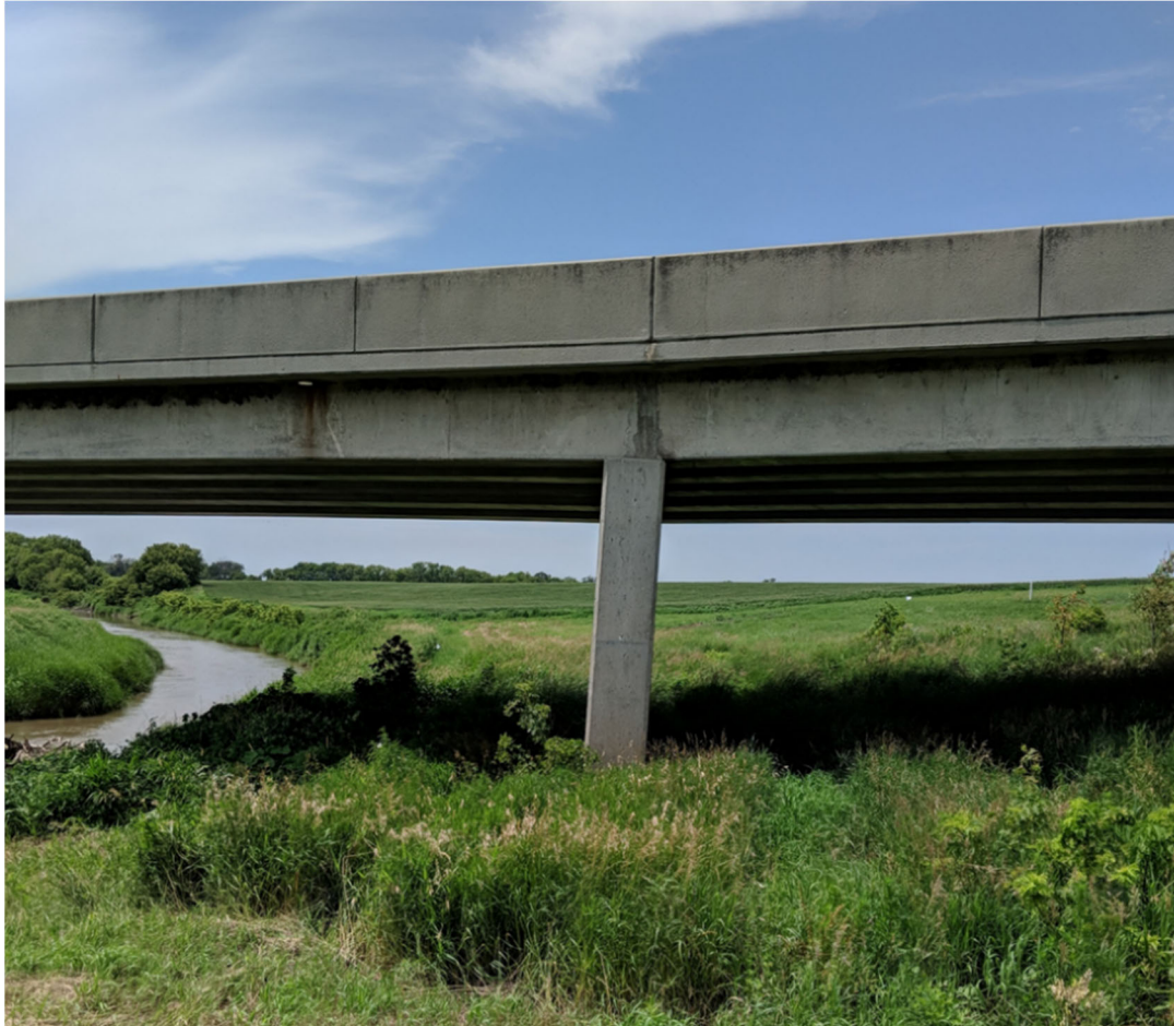
Figure 2 – North Pier Leaning from Landslide
